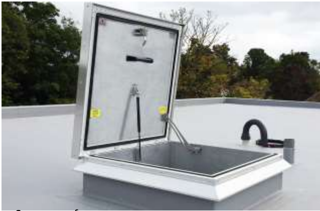
Secure roof access
